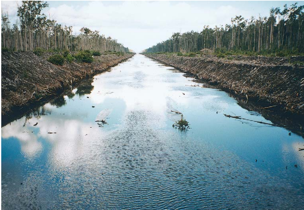
Mega Rice project drainage and irrigation channel in 1999, excavated along a tropical peatland watershed in Central Kalimantan, Indonesia. Photo: Jack Rieley & Susan Page. (§ 3.4.1 (ea))
