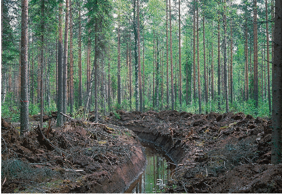
Recently excavated ditch in peat soil. Mixed tree stand (Pinus sylvestris, Betula pubescens and Picea abies), Southern Finland. Photo: Juhani Päivänen. (§ 3.4.1 (eb))
