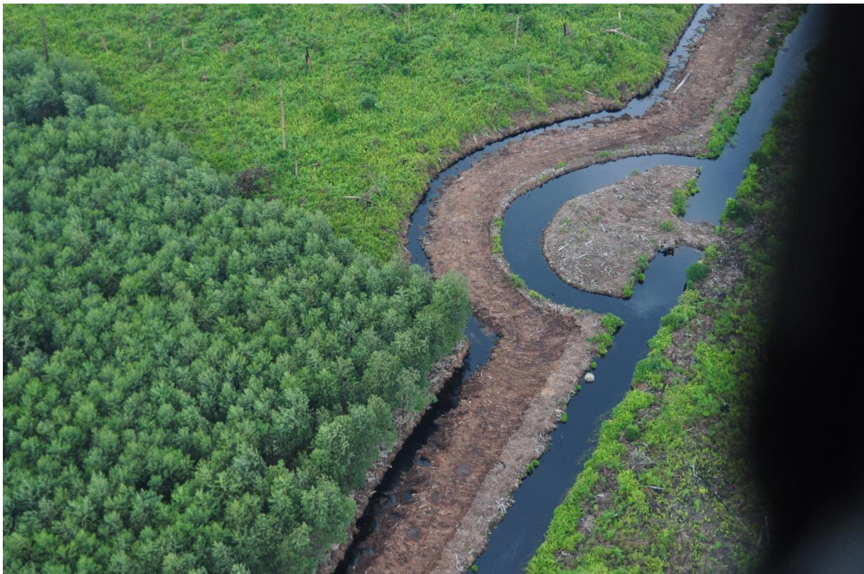
Dam construction in APP acacia plantation in Jambi, Sumatra. Photo: Hans Joosten.
