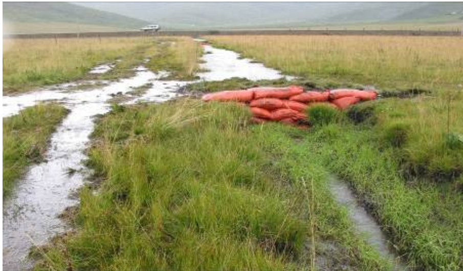
Fig. 46: Successful rewetting by a small dam made of plastic bags, filled with sand
