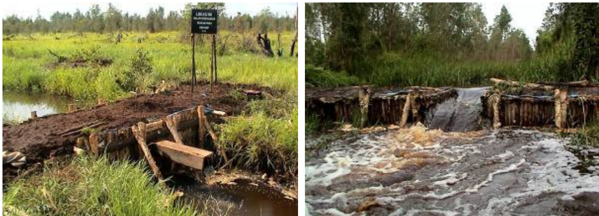
Fig. 28: Small dams made of wood, plastic and peat (blocking canals of 1 – 3 m width)
