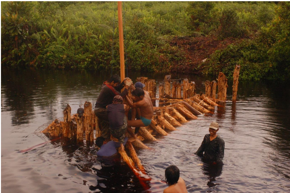
Manually building dams in a peatland drainage canal in Central Kalimantan, Indonesia. Photo: Hans Joosten.
